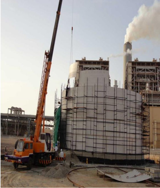
Co2 Piping, SS piping, Structural works, GRP lamination and piping – Shuaibah III
